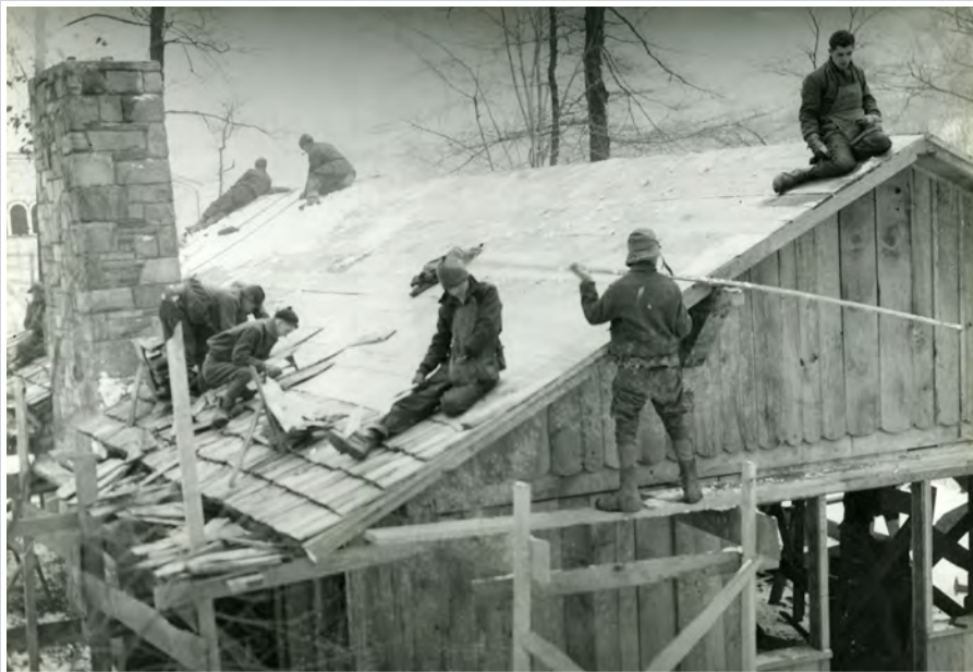
February 1937 Construction workers employed by the Civilian Conservation Corps built a shelter at Gorge Metro Park within a week.
